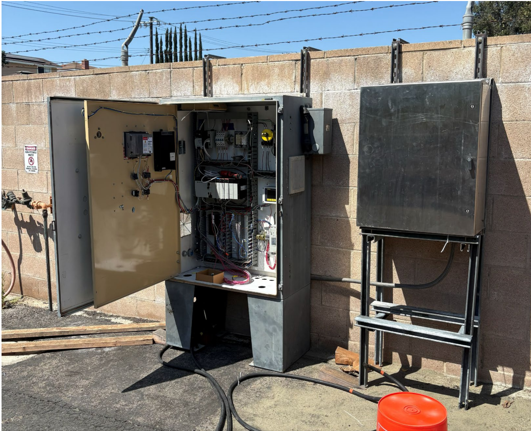
Figure 3 –Temporary Power Panels at Freeway Lift Station
