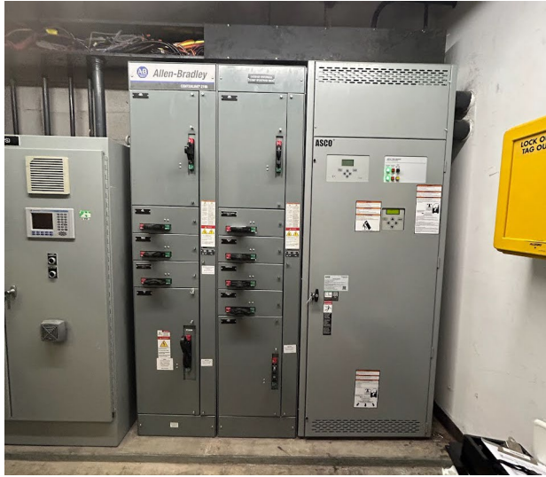
Figure 1 – New Automatic Transfer Switch and Switchgear Panels
