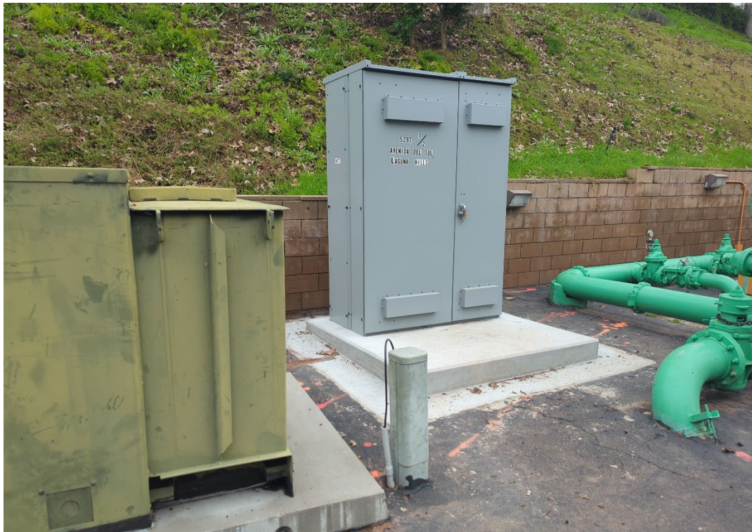
Figure 3 – New Main Switchboard
