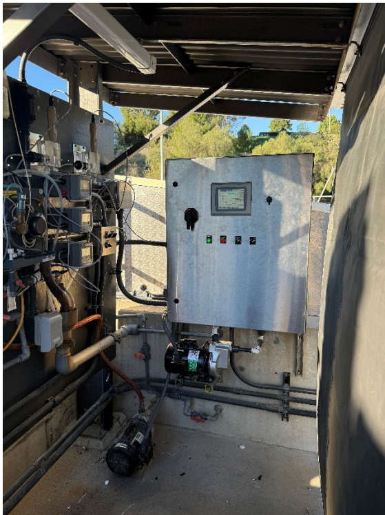
Figure 1 – New Local Control Panel for Free Chlorine Disinfection
