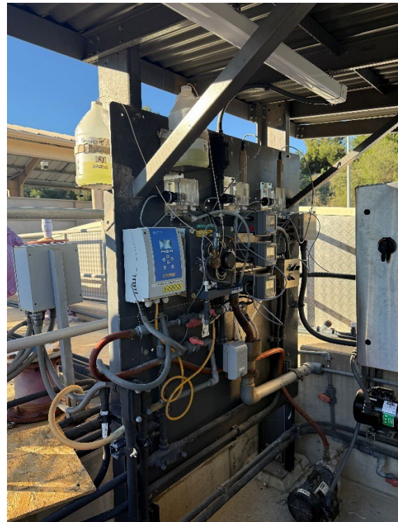
Figure 2 – New Free Chlorine Disinfection Analyzer Panel
