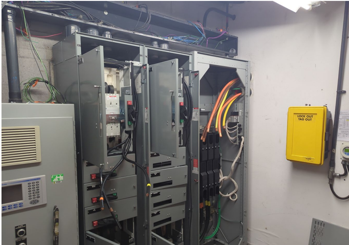
Figure 4 – New Automatic Transfer Switch and Switchgear Panels
