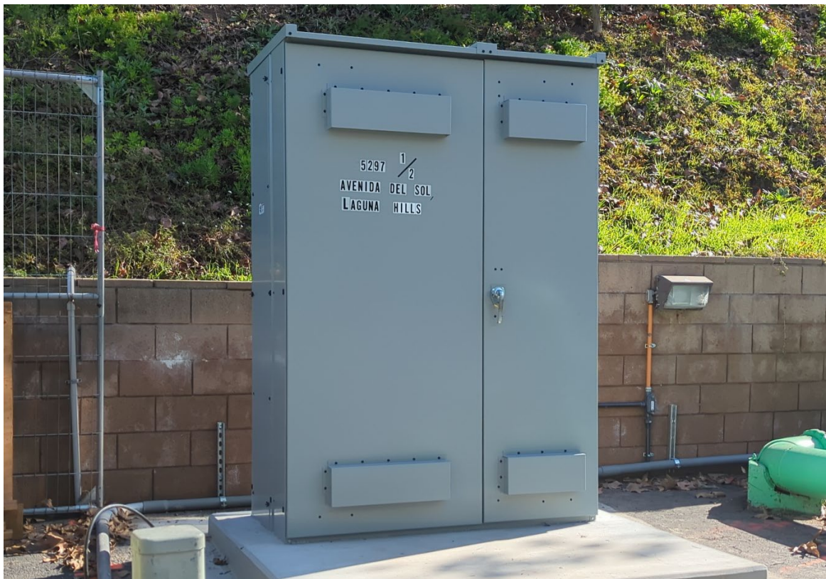
Figure 1 – New Main Switchboard
