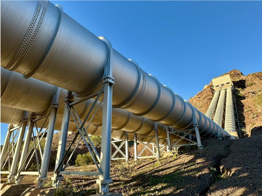
Gene Pumping Plant
