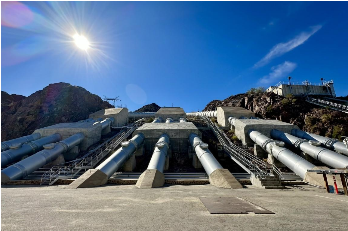
Whitsett Pumping Plant
