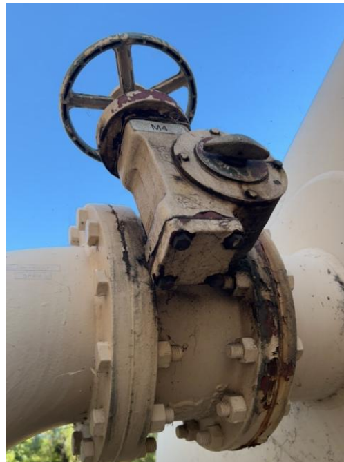
Figure 2 – OOPS Surge Tank Isolation Valve
