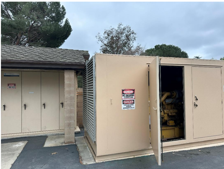
Figure 1 – Westline Lift Station Generator
