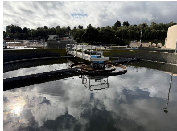
Figure 6 – Secondary Clarifier No. 4
