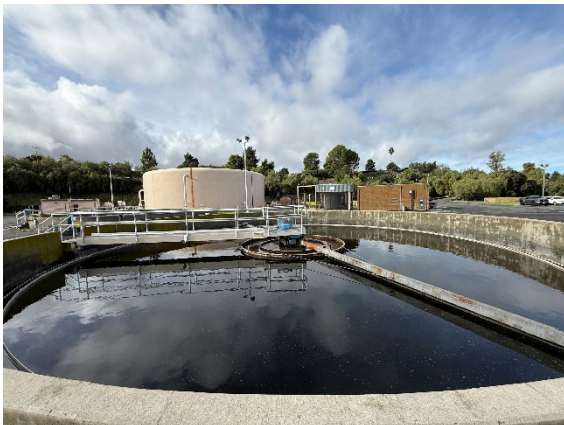
Figure 5 – Secondary Clarifier No. 4
