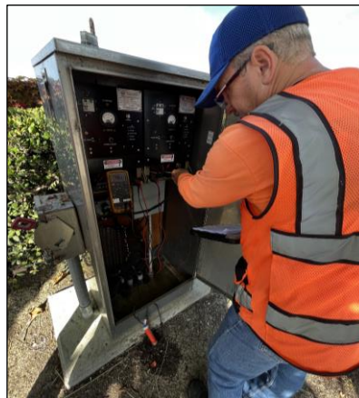
Figure 1 – Typical Rectifier Testing/Inspection
