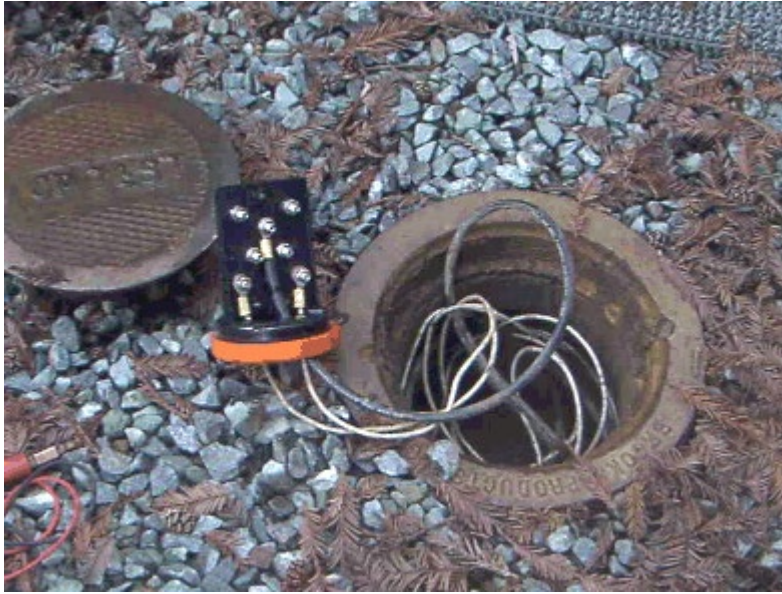
Figure 2 – Example Test Station in Valve Can
